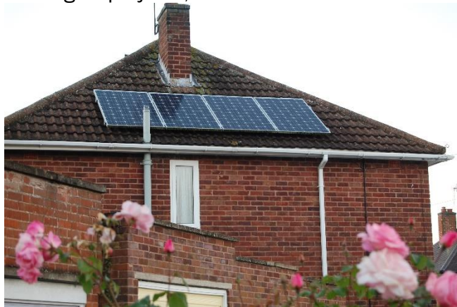
FIGURE 19: DOMESTIC PV PANELS
